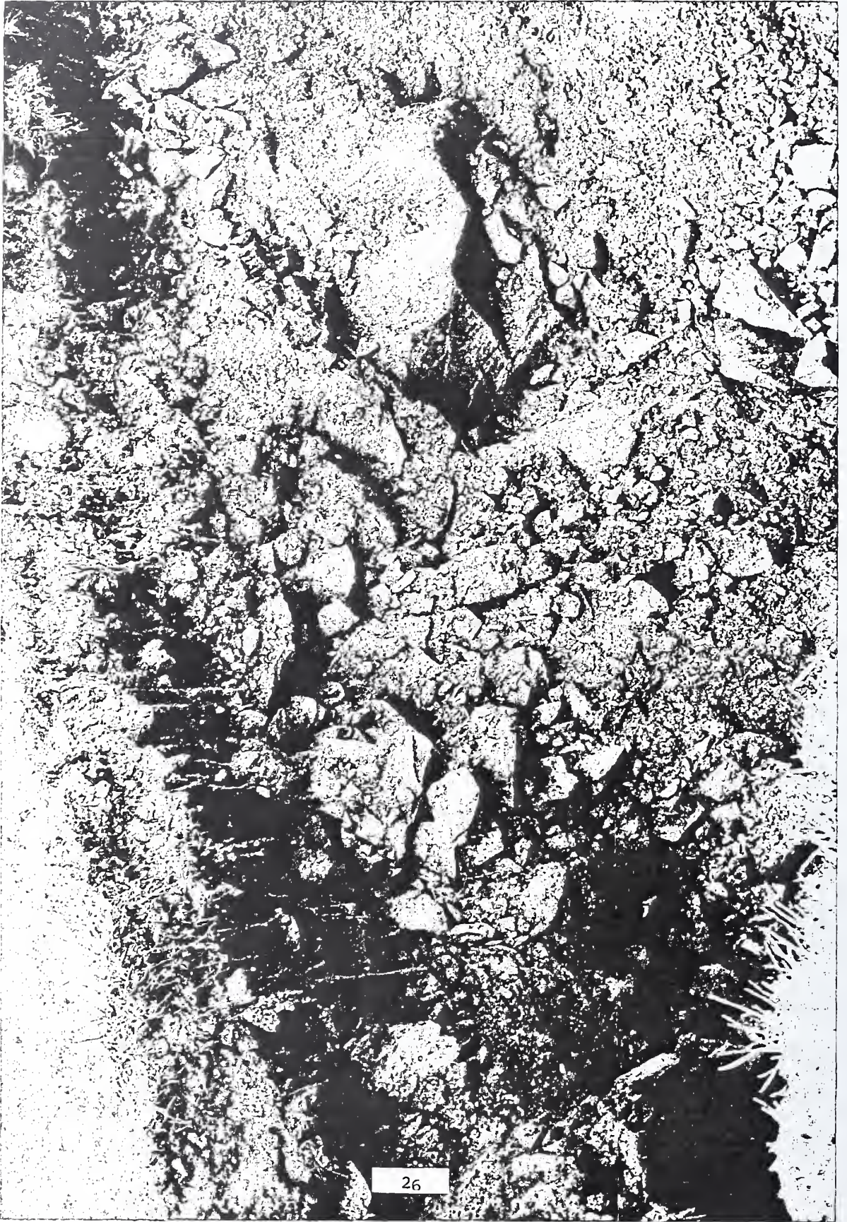
Figure 9. Rock rubble in the water and sewer service trench at 4909.
